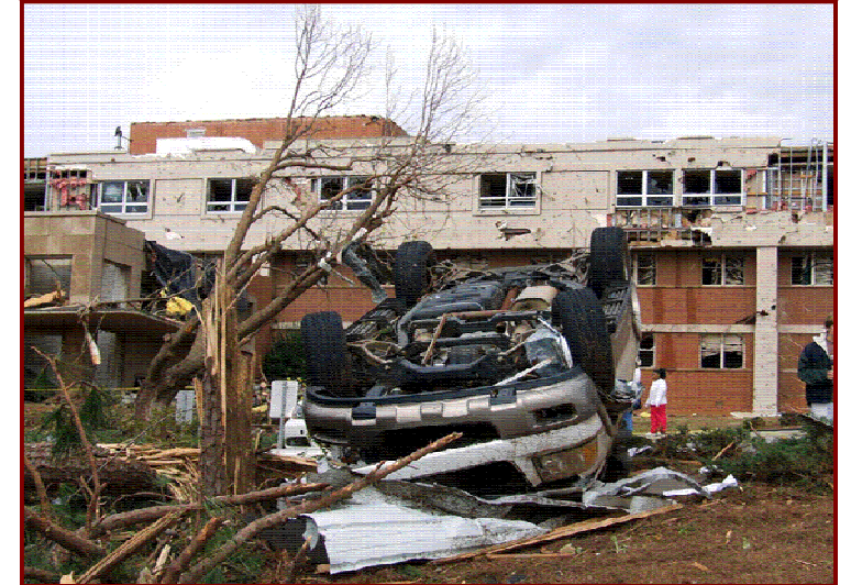
A tornado struck Sumter Regional Hospital, Americus, Georgia, after 9 PM on March 1, 2007. 55–60 patients were evacuated, but damages were so extensive the hospital later had to be razed.
